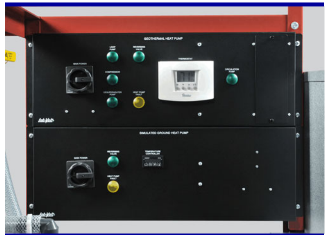
Geothermal Heat Pump control panel and Simulated Ground Heat Pump control panel.
