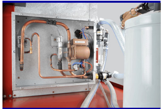
Partial view of the domestic hot water system.
