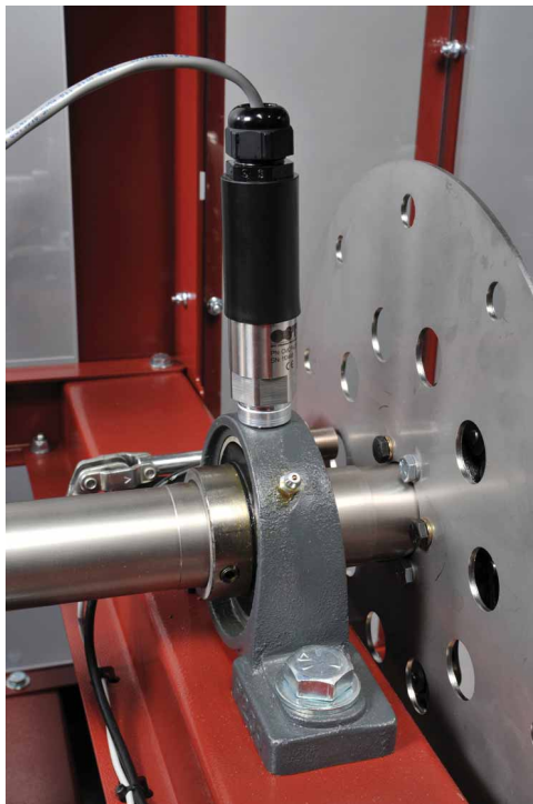
Figure 2-35. Vibration sensor on the pillow block.
